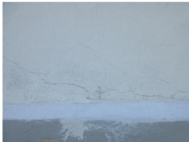
Sprickor i fasadens puts.
